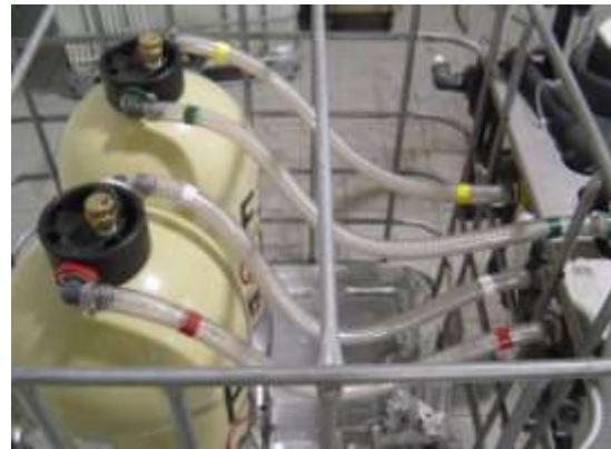
Figure 26: Rear View of Valve Assembly, F1, and F2 Hose Connections
