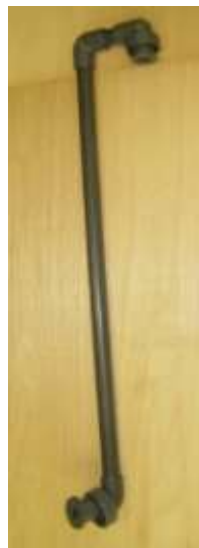
Figure 20: Tablet Chlorinator Feed Line
