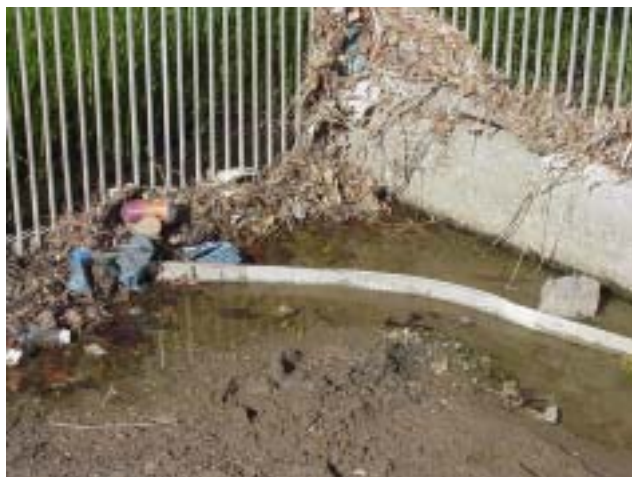
Figure 7 Site 10 cement drain with barrier and rubbish build up
