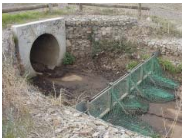
Figure 9 Site 14 cement drain with gross pollutant trap
