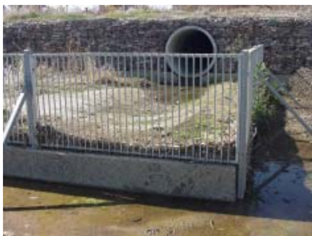
Figure 8 Site 11 cement drain, showing build up of silt/dirt
